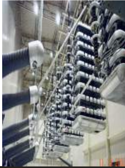
Thyristor Valve HVDC Classic
