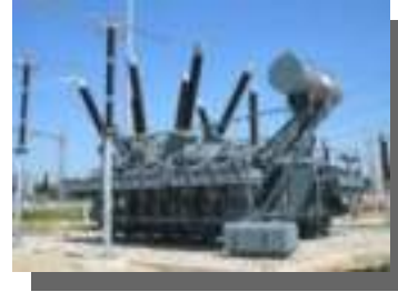
Phase Shifting Transformers
